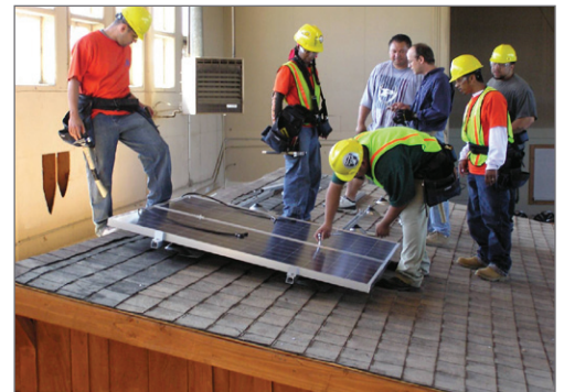
Richmond Works YouthBuild students learn to connect solar panels to a roof in a warehouse sized classroom model, partnering with their local utility. (Richmond, CA)
